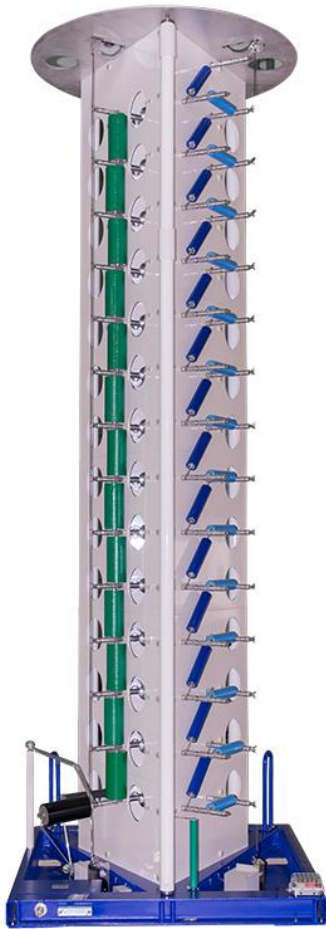
1400 kV Impulse Voltage Generator
