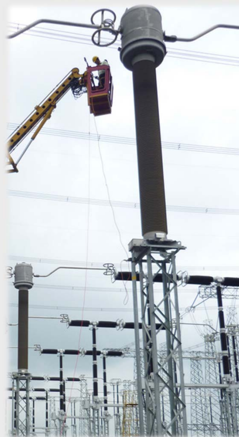
India 765 kV substation
