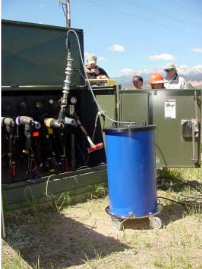
Coil / HV Switch / PD detection circuit
